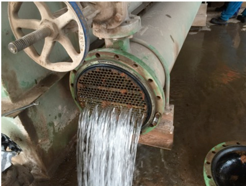
Heat exchanger after installation 2 months
